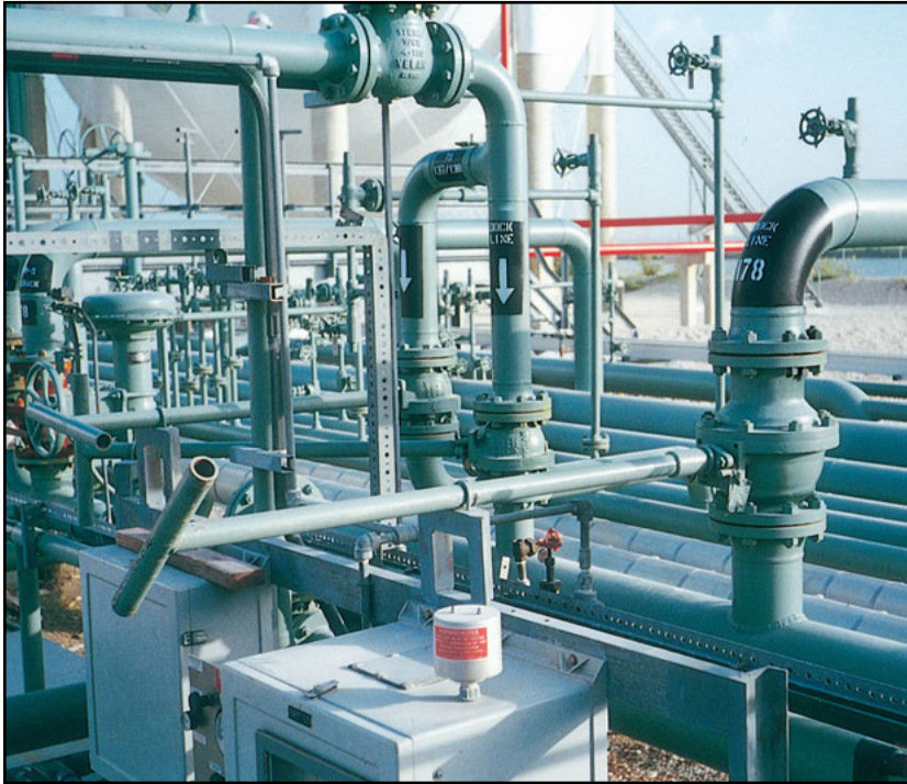
Installation of NPS 6 (DN 150) SB-150 with extension handle at a Texas refinery.
