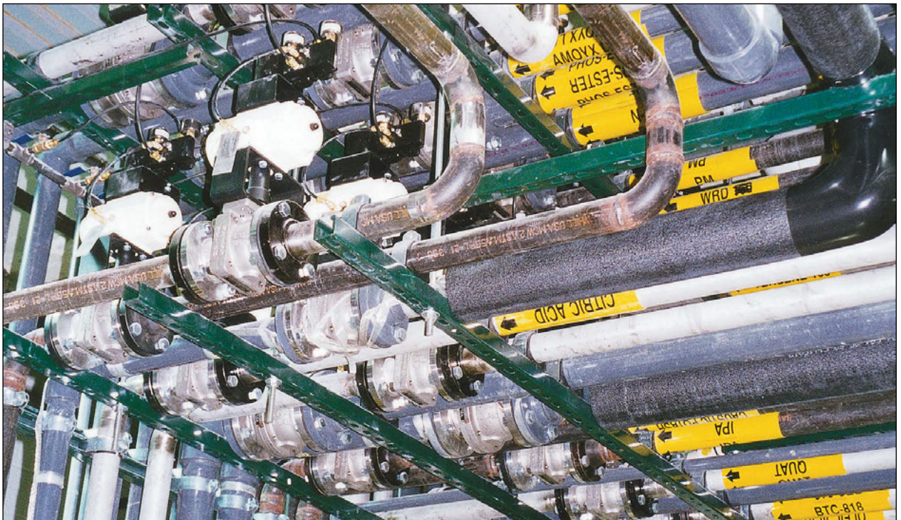
Split-body ball valves installed in a chemical plant in Ohio.
