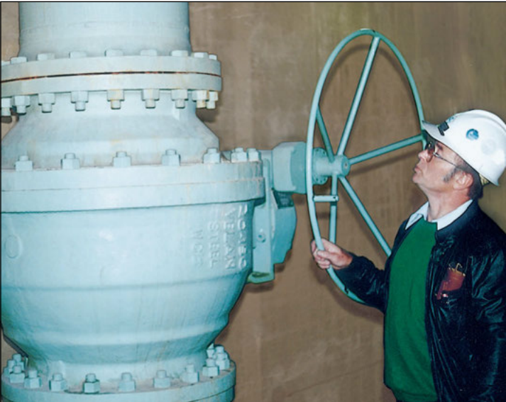
NPS 20 (DN 500) split-body bypass ball valve installed at James Bay in Canada.
