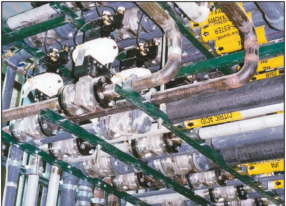
Velan split-body automated ball valves sizes NPS ½ – 4 (DN 15–100) installed in a major chemical plant, in Ohio.
