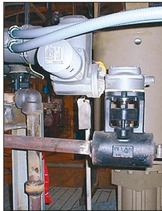
A Velan Power Ball valve in high-pressure steam service.
