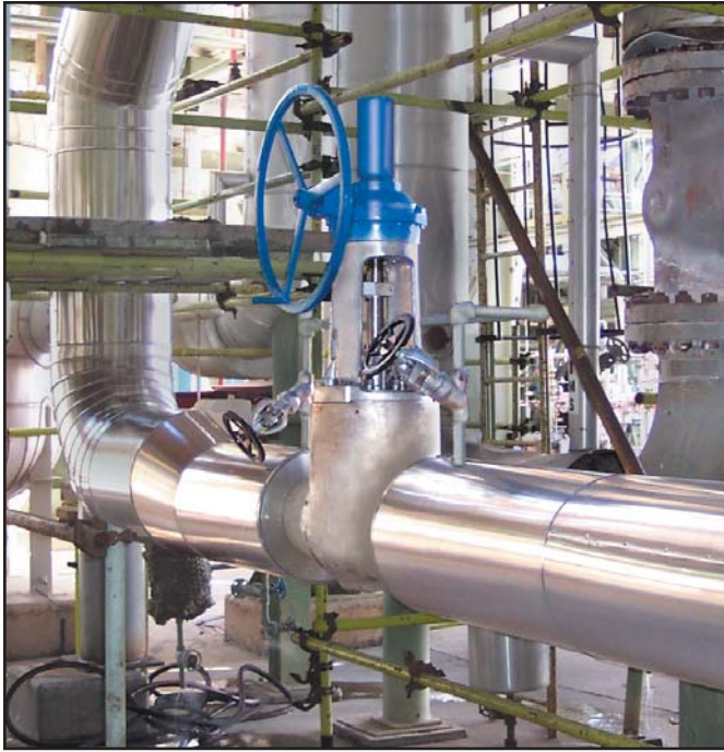
10" (250 mm) Pressure seal valve installed at Profertil's plant in Bahia Blanca, Argentina.
